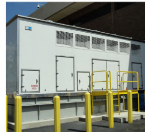
DEDICATED GRID STATION
